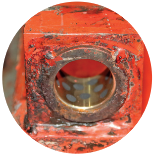
④ Lower bearing modified from DU plain bearing bush to solid bronze bush with solid lubricant
